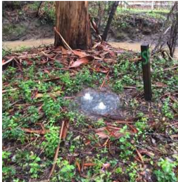
(Example of overflowing manhole)
