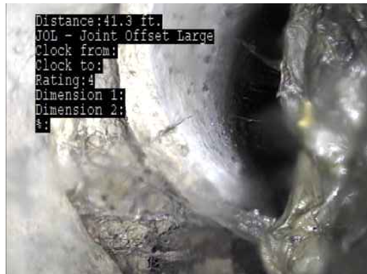
① LARGE JOINT OFFSET USMH K11146 TO DSMH K11132 SCALE: NO SCALE
