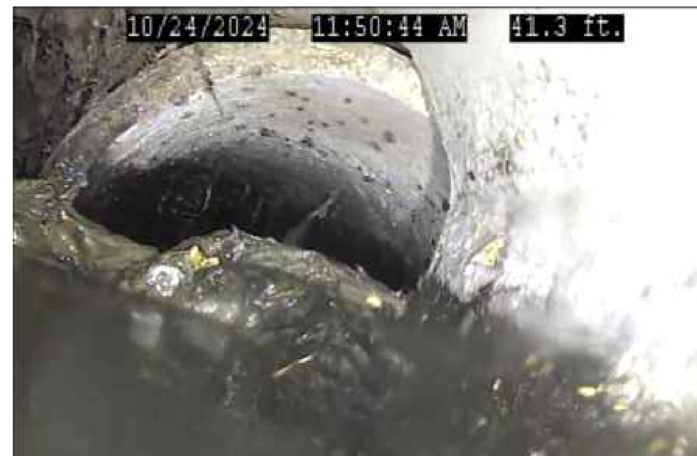
② SURVEY INCOMPLETE DUE TO BLOCKAGE USMH K11146 TO DSMH K11132 SCALE: NO SCALE
