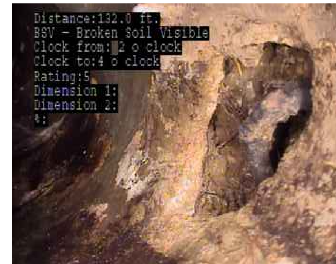
⑥ BROKEN PIPE LEAVING SOIL VISIBLE USMH K11144 TO DSMH K11145 SCALE: NO SCALE
