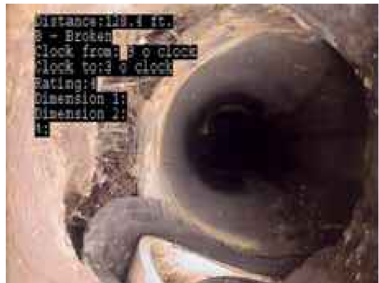
④ BROKEN PIPE LEAVING LARGE JOINT OFFSET USMH K11144 TO DSMH K11145 SCALE: NO SCALE
