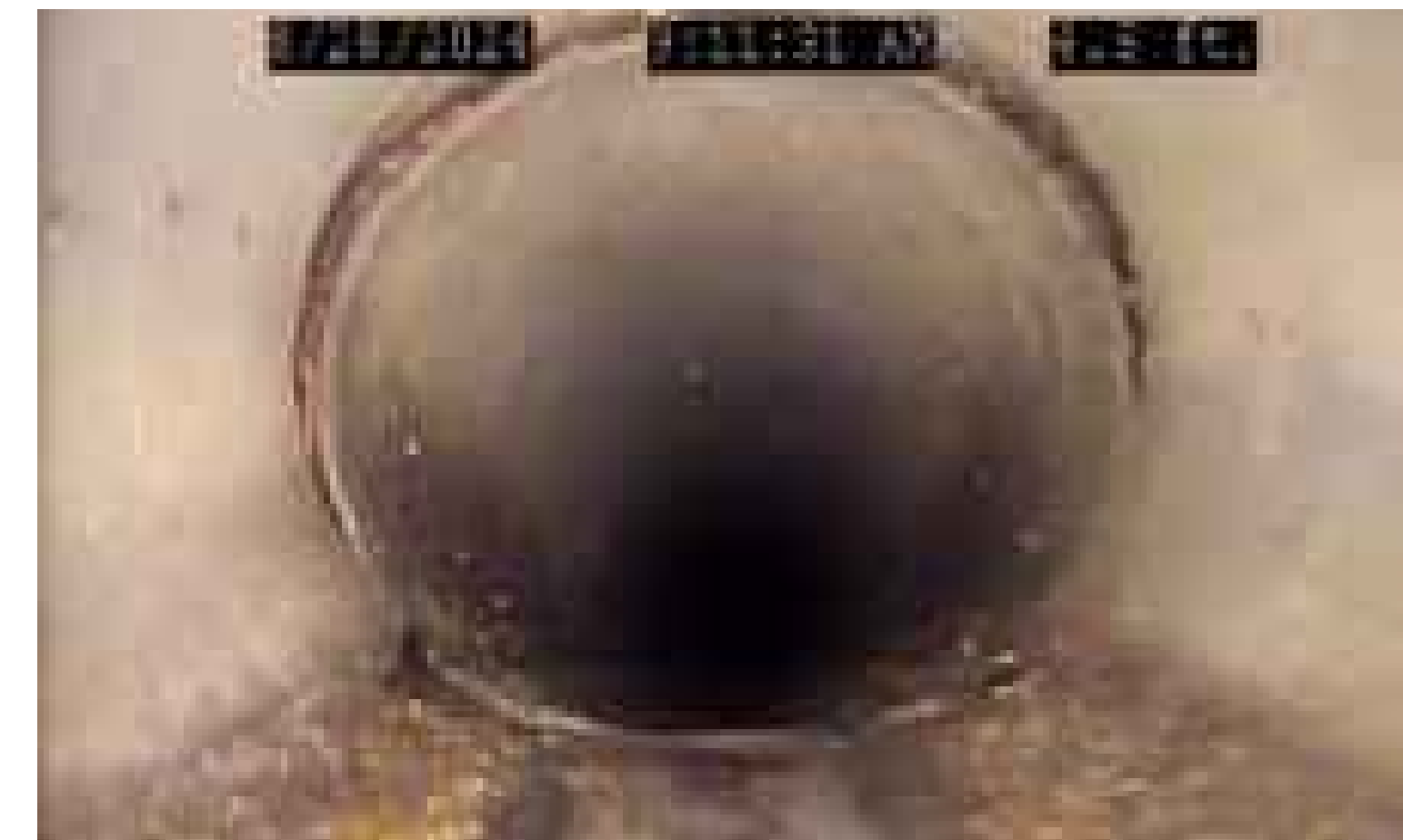
③ VERTICAL DEFLECTION, PIPE ALIGNMENT DOWN USMH K11145 TO DSMH K11146 SCALE: NO SCALE
