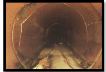
Cracked Clay Sewer Pipe
